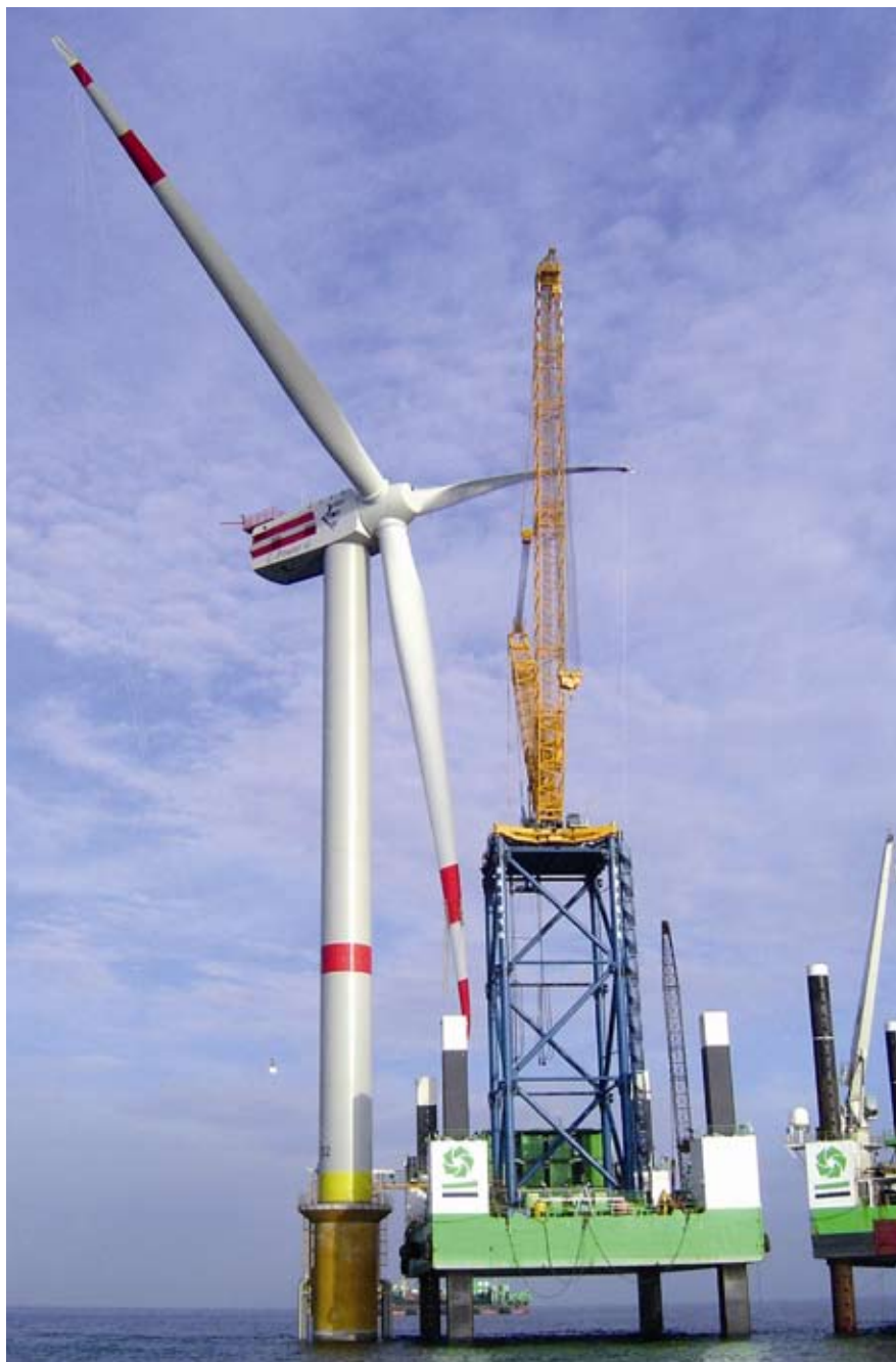
The first six turbines installed completed the first phase of the Belgian Thornton Bank project in September 2008. Picture: Jan Oelker
