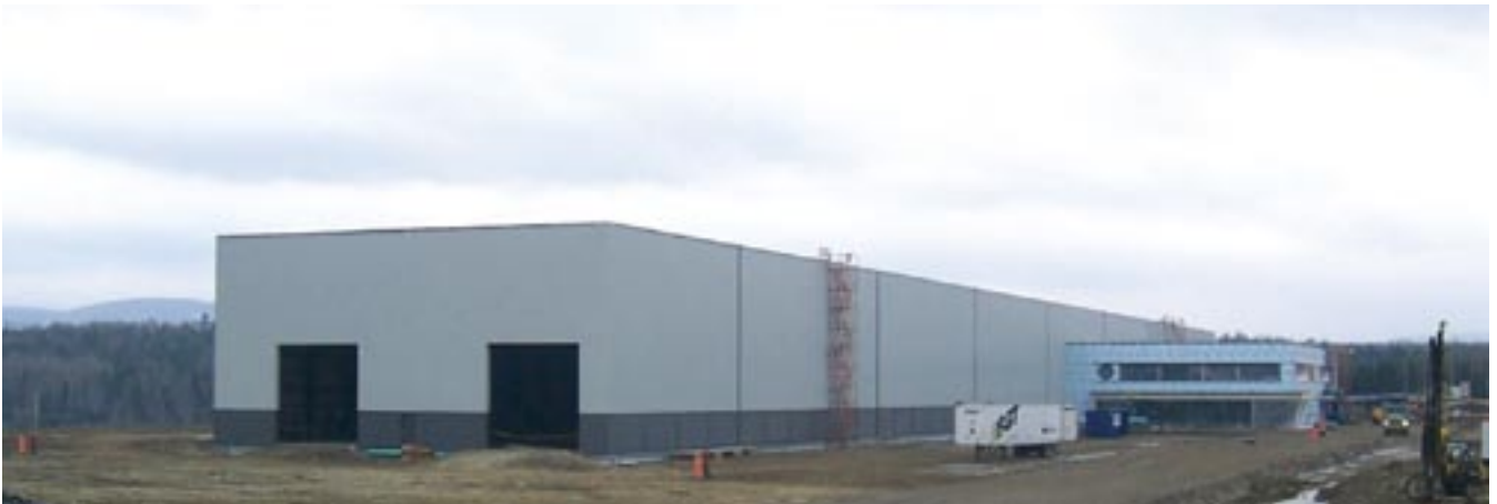
The factory in Gaspé, Canada, will be ready for production by January 2006. Construction of this factory, located in a new industrial area on the outskirts of the town, has taken approximately 6 months.
