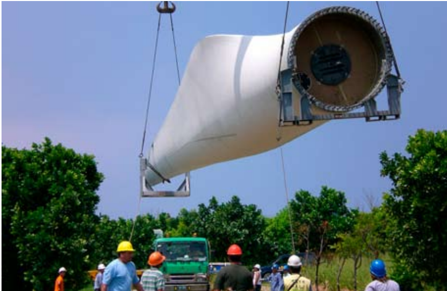
A blade is being lifted by crane to the truck, which will take it to the workshop.
